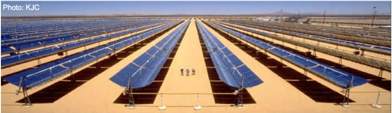
Figure: Kramer Junction California Solar Thermal Power Plant
